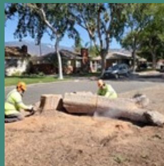
Crews removed a hazardous tree on W. Bernard Way (Ward 2)
